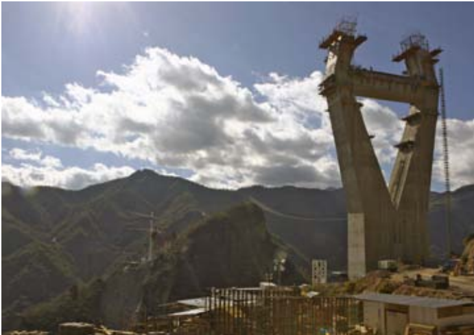
Mexico's Baluarte Bridge is currently under construction. When completed, it will be the longest, highest cable-stayed bridge in all of Latin America.
